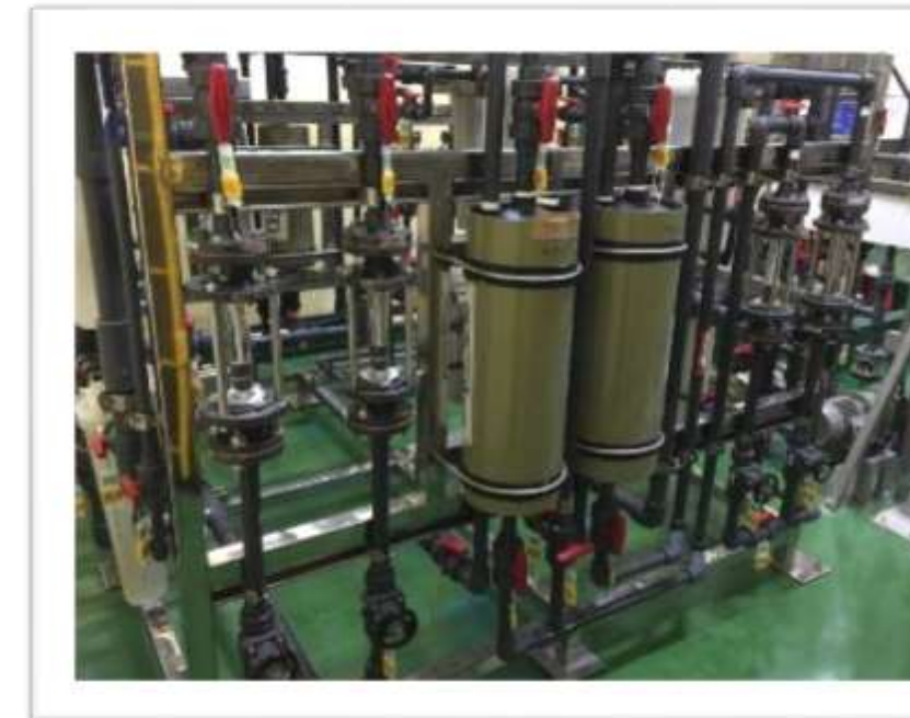
NH 3 Membrane separation unit
