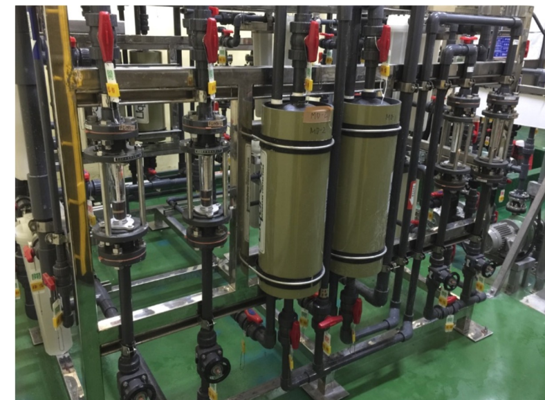
NH 3 Membrane separation unit
